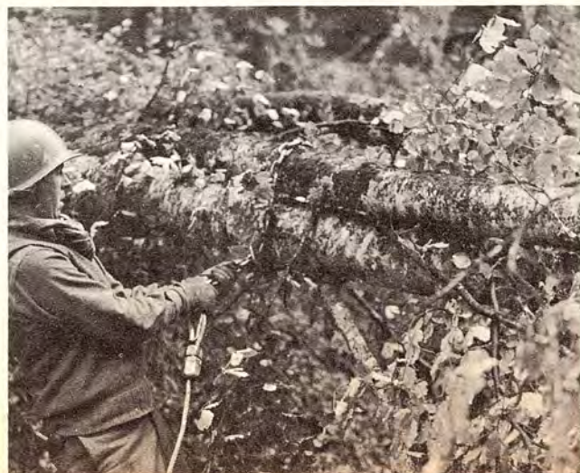
ENGINEER HOOKS CHAIN AND CABLE AROUND TREE TO BE PULLED FROM ROADBLOCK.
