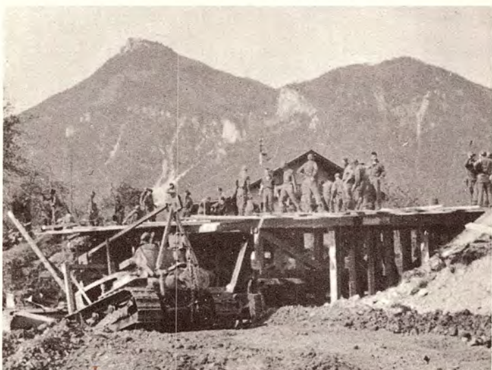
LAST SPAN: Engineers opened the road to Kufstein with speedy timber-trestle construction after Germans had blown bridge.
