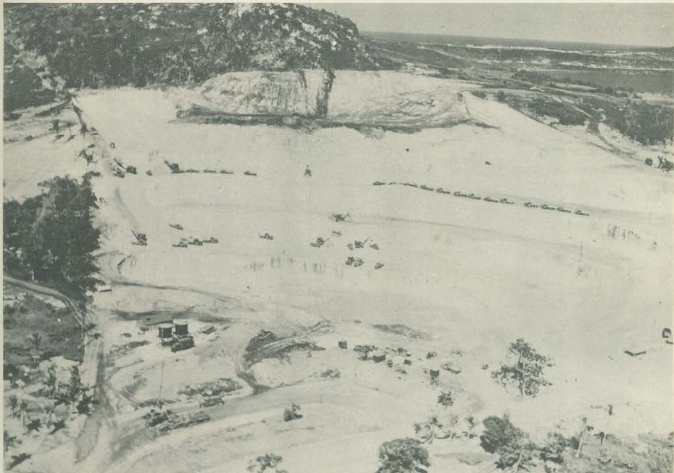
One truck every forty seconds moves out of the enormous quarry carrying coral to surface strips
