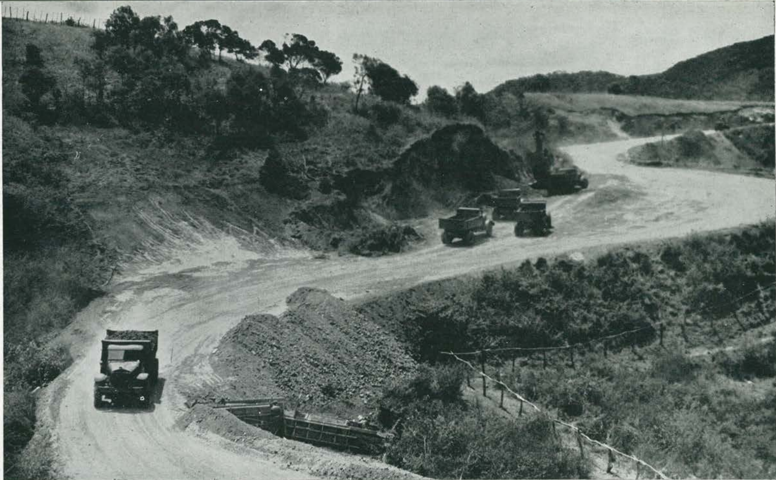
LITTLE BURMA ROAD. Snaking over exceedingly treacherous mountain passes, the original road above Bourail was actually no more than a narrow 15-foot wagon trail. Earth, cut away from the bordering red-dirt bluffs, was dumped over edge on opposite side
