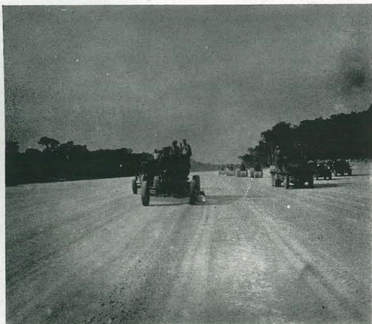
PERFECT FORMATION. Tandem lines of graders and rollers are shown during "face-lifting" operation performed on Stirling Field runway early in June. Harvil Nolin and George Sembrat, equipment operators, are leading grader parade. Work was continuous for two days and nights.
