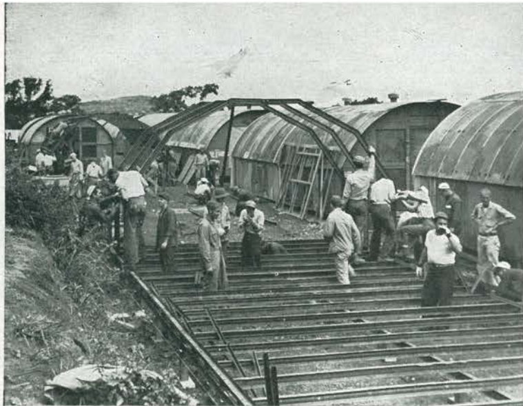
ASSEMBLY LINE. Four quonsets every eight hours was the record set by the four carpenter crews of 10 men each. Here, Chief Sam Beacom stands by as the arches are being hoisted into place on the steel-ribbed foundation.
