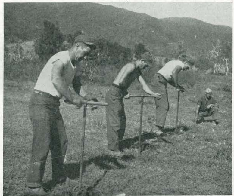
HEAVE HO! Miles of fence had to be reset by hand to make room for the road widening. Chief Al Broomfield (right) directs a straight line for the post-hole diggers, who are (left to right): Listenberger, Perlak and Ahlf.
