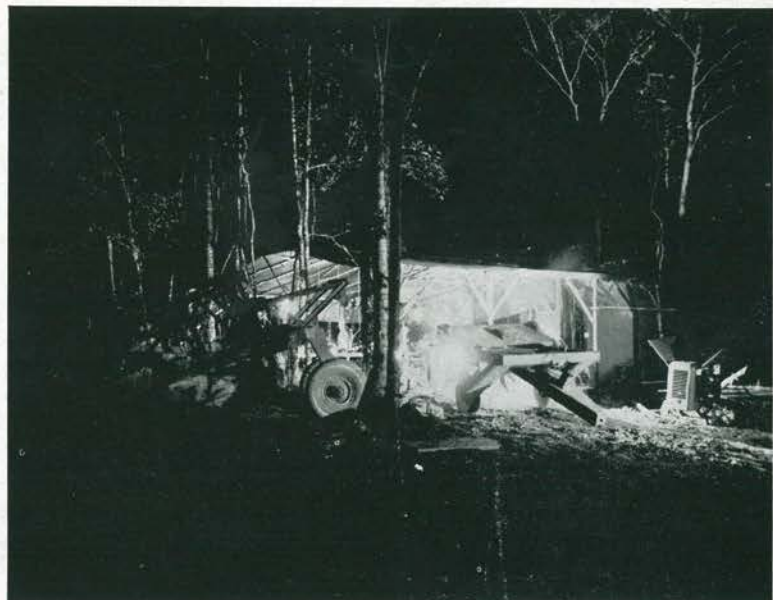
CASUALTIES. The welding shop was part of the equipment "sick bay." The going was tough and it wasn't always the coral that moved. A pan pulled out of shape and a rooster hitch pulled apart are being "treated" by welders.
