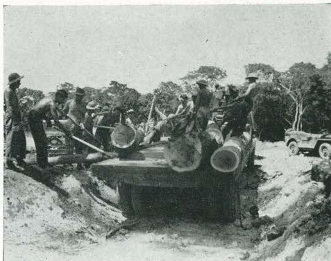
AND THEY CARRIED THEM AWAY TO THE MILL. Lumber for pilot housing was sawed from timber cleared from the Strip. Here, Bos'n's Mate Meredith Walls and crew load out a few. A 'dozer ditch accommodates the trucks and eliminates uphill pull.
