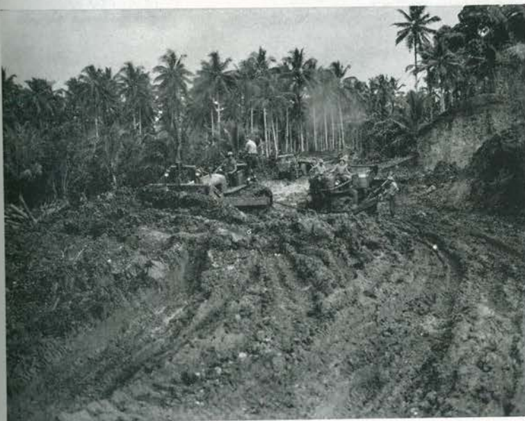
MUD. Even giant bulldozers sometimes bog down in tropical mire. Here, Tom Hutson rescues "Chet" Wlostoski and his stuck 'dozer from the muck. Huge fills in swamp made this road project a stiff proving ground for both men and equipment.
