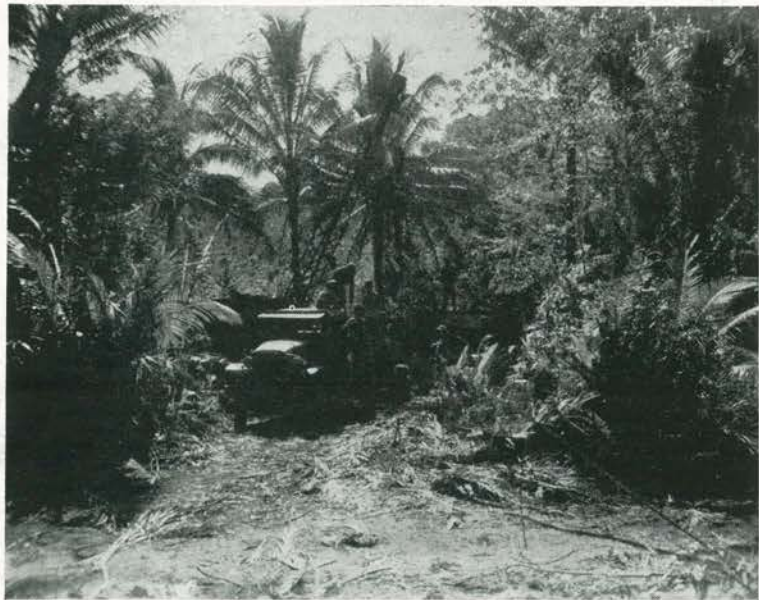
HIDEAWAY. Surrounded entirely by tangled vegetation, cleverly camouflaged by Nature, a back-saving crane assists battalion storekeepers and riggers laboriously unloading pallets of invaluable supplies from ships to be hidden in this secret supply dump.
