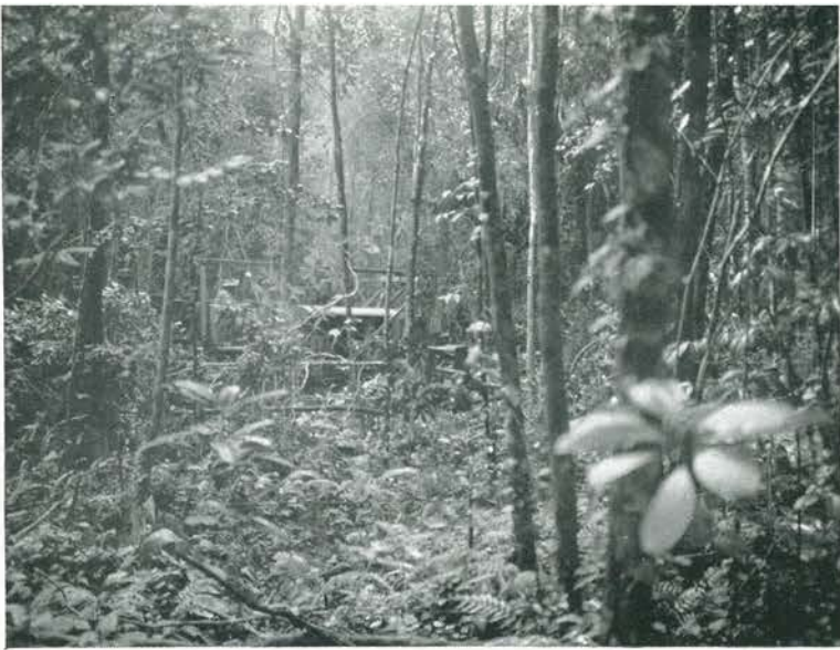
LET THERE BE LIGHT! This isn't a night clearing scene. It was just this dark when the first bulldozer arrived on the centerline of Stirling Strip the first morning of clearing operations. Lights were soon installed in the virgin jungle.
