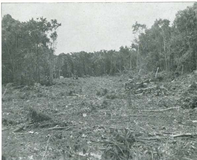
AND DAY IS DONE. The end of the first day. An area of 300 feet in width and 600 feet in length has been roughed clear. A good, fast start on a good fast job—on the road to Tokyo! However, the 87th was to build many more strips before V-J Day.
