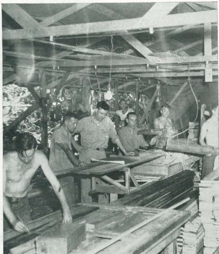
CARPENTER SHOP. Chief Carpenter's Mate "Bob" Parrott and Carpenter Karl Jchannessen (left center) study detailed blueprint at an improvised table while machine-handy assistants turn out all types of furniture from native lumber for the 87th and other units.
