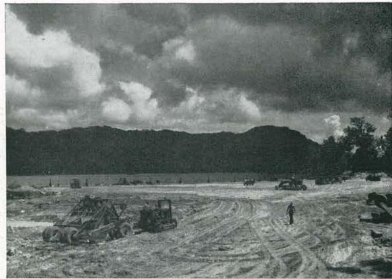
HILL DISAPPEARS. Grading of the cleared dock area is now progressing by leaps and bounds. The hill, which formerly was here, has been carved away and used as fill on shore access road. Plane tender is anchored offshore with PBVs.
