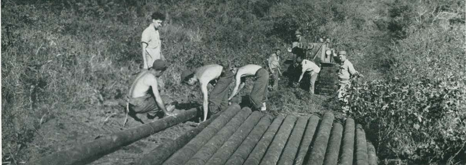
WATER MAIN. Laying the principal waterline into the Monte D'Or camp involved skinning the heavy pipe a distance of approximately two miles over the rolling, scrubby hills adjacent the towering mountain range. An
