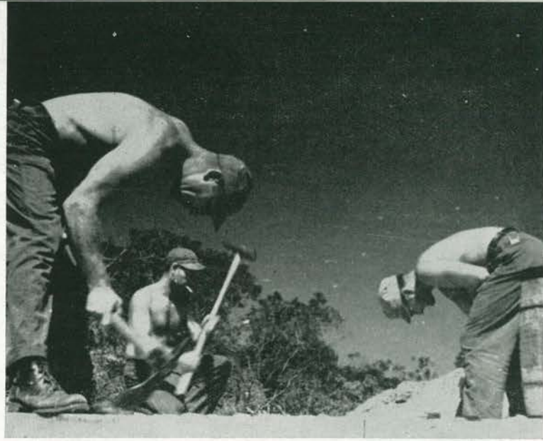
SMOOTHIES. Final touch to the bridge was smoothing off rough, uneven planking and rounding off end approaches. Here, men revert to use of time-honored adze, which in hands of such men as Gordon, Lingle and others, gets results.
