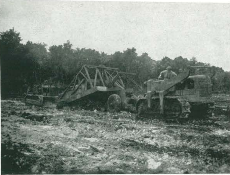
SKIMMING OFF THE MUD. Before grading the runway to shape, it was necessary to clear off the black humus overburden. Here, two HD-10s struggle to load an eight-yard pan with the sticky muck shortly after a terrific downpour.
