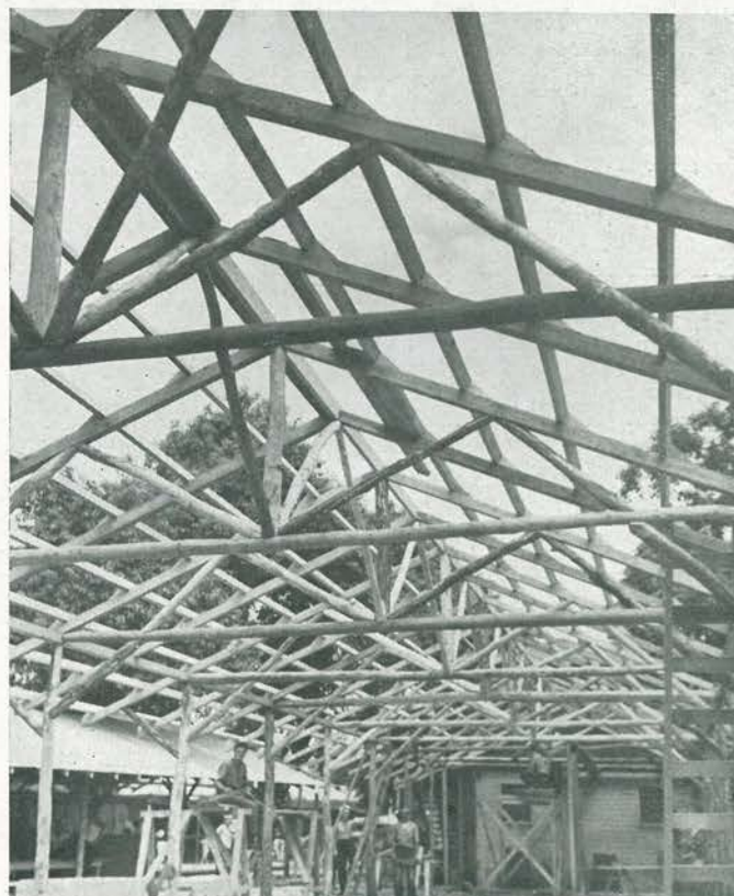
RUSTIC UPHOLSTERY. Framework for all structural work in compound was of native rough timber and a minimum of finished lumber. Project was stymied time and again for lack of sufficient building materials. Here, construction was still in progress.
