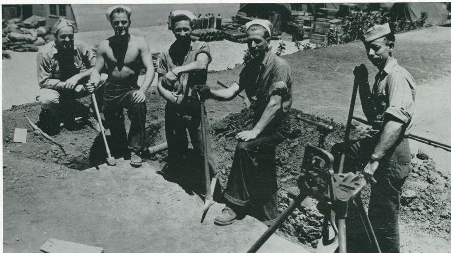
NOT IN THE CONTRACT. Battalion plumbers were truly "jacks-of-all-trades." Besides piping the entire camp for showers and plumbing Sick Bay, mess hall, laundry, etc., they frequently had to dig their own ditches
