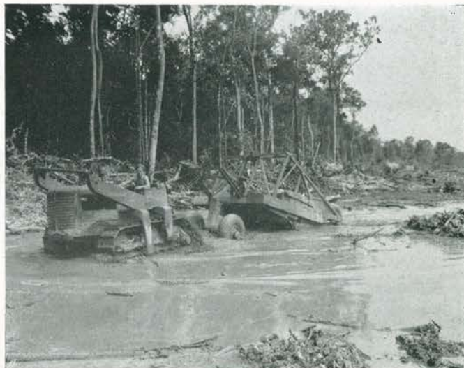
COME HELL OR HIGH WATER, the gang was in there pitching. Frequent cloudbursts were a considerable inconvenience, but work continued just the same. That glum look on Clyde Pemberton's face is probably the result of a very damp "driff."
