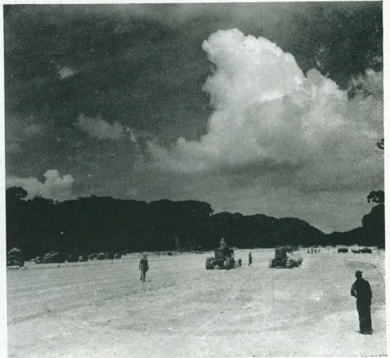
TAKING SHAPE. While pans are bringing the section to close rough grade (left), the grader is working the finish (right). Up ahead can be seen the demolition and donicker removal crew. (See page LXIII of CAN DO.)
