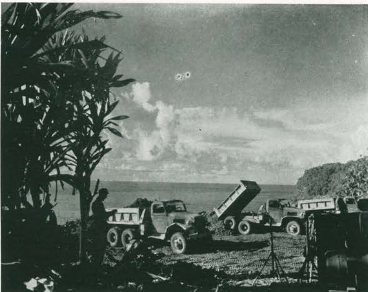
GETTING RID OF IT FOR KEEPS. Gushion E. Bolt supervises from the shade of a convenient tree as trucks dump loads of strippings into the sea some 80 feet below. Most stumps and roots were disposed of in this manner—once and forever.
