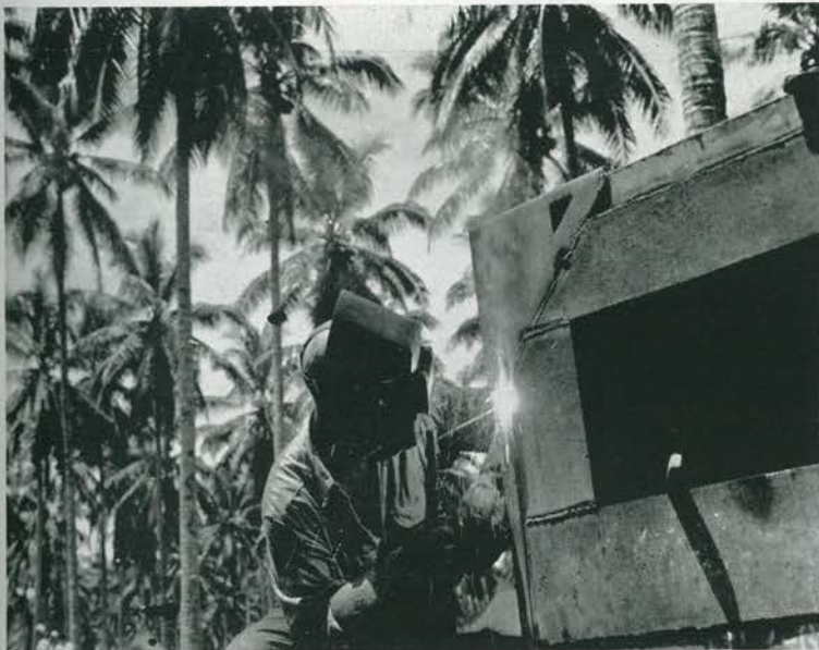
ON TARGET. Vernon Jacobson welds on a section of pontoon. Seabees had put pontoons to many ingenious uses, but none more unusual than this unit. Upon completion, this one will serve as an oven for the bakers.
