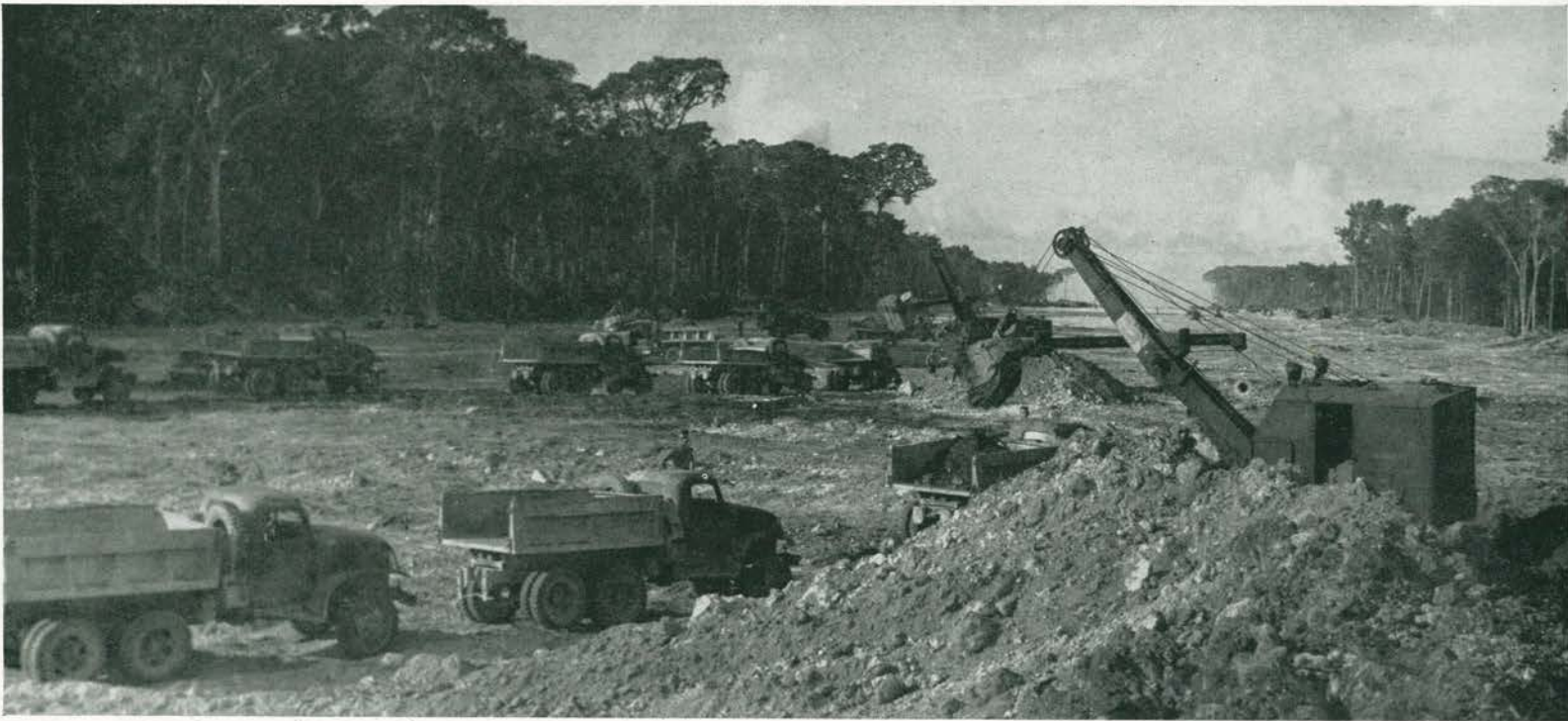
EARTHMOVERS EXTRAORDINARY. In foreground, bulldozers have pushed waste humus material into large piles from which three-quarter shovels are loading trucks. Further back (left), pans are engaged in final stripping. A group of pans (background) are cutting and filling coral, bringing the
