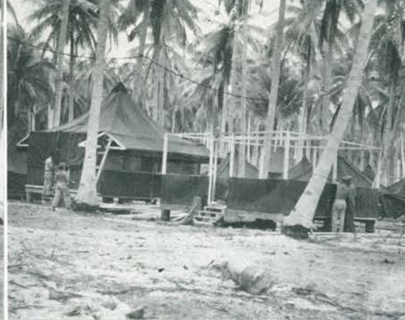
Tents under construction. Coconut logs cut in our own sawmill furnished lumber for framing.
