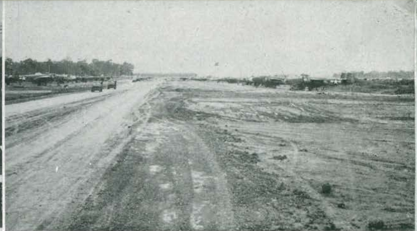
A part of the taxiway and parking area at Palawan. It took weeks of work by the Seabees before things looked like this.
