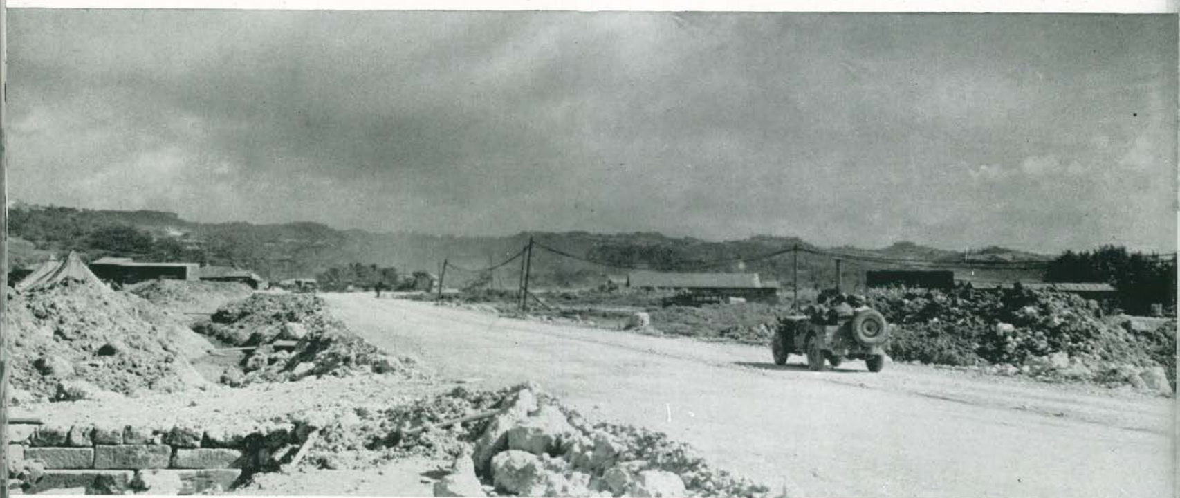
Top: A bulldozer and dragline filled in the last section of Highway 13 on which Blackjacks worked Bottom: When the weather dried up a little, Highway 13 had a solid coral base and surface
