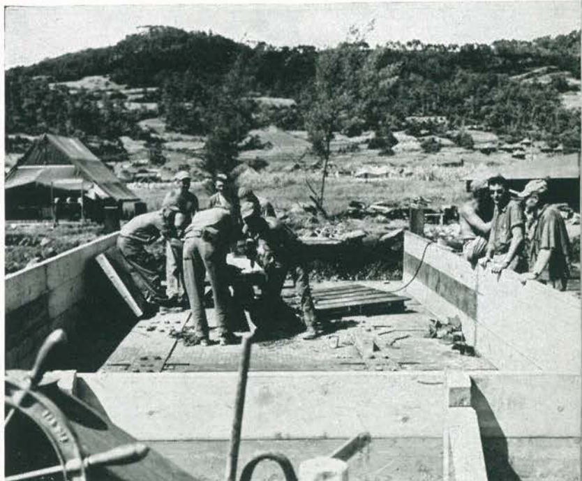
Top: Seventeen acres were cleared and graded for the 17th Seabee Regiment dump.
