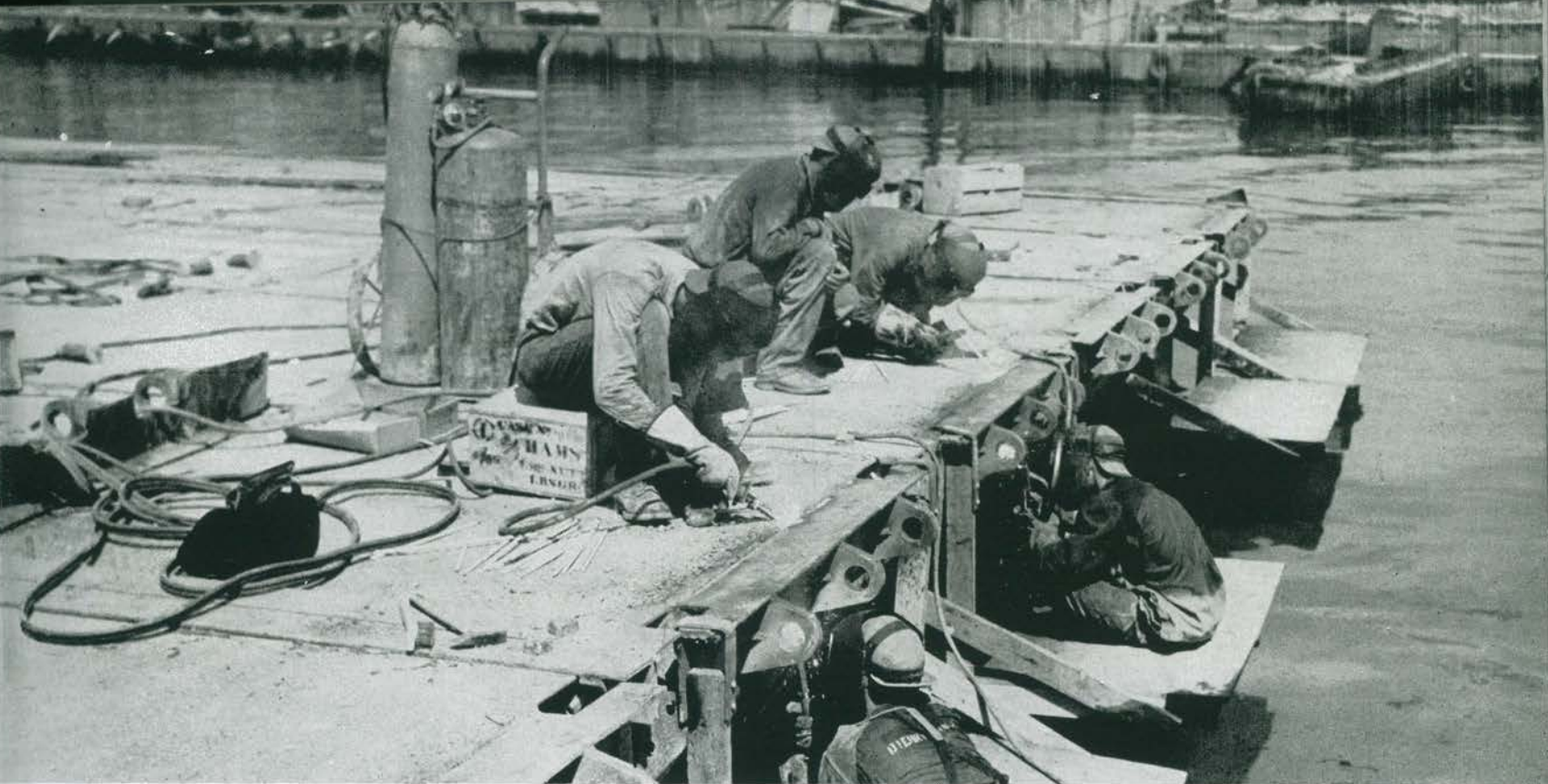
The pontoon sections were held together by hinges which were welded to the sides
