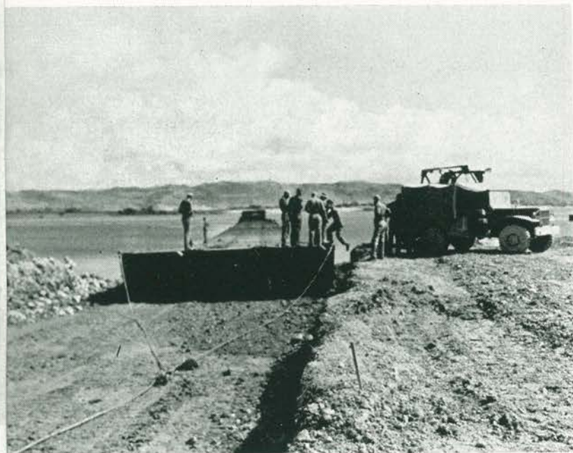
One end of the pontoon assembly was pulled ashore by a "cat"
