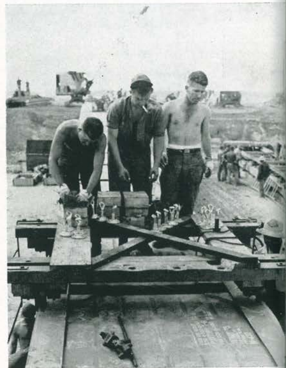
Stokey, Stackhouse and Sharp set up the "Toonerville Trolley" which Sharpe had designed to reduce assembly time 20 percent.
