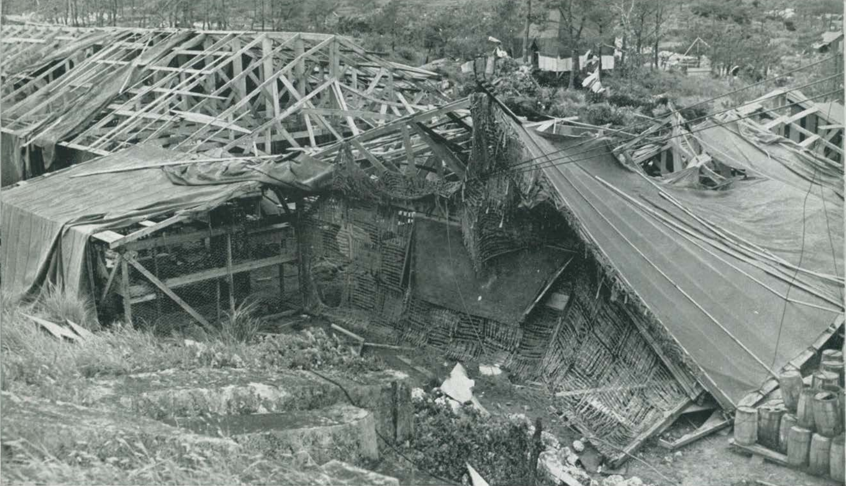
The carpentry shop was smashed, as were the heavy equipment repair and transportation shops
