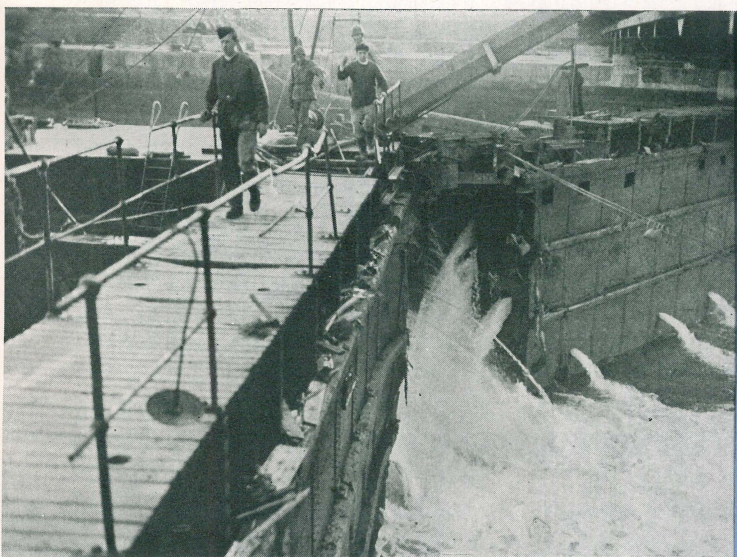
The Rochemont lock, key to Le Havre's inner basin system, was bulldozed into operation by Army engineers.
