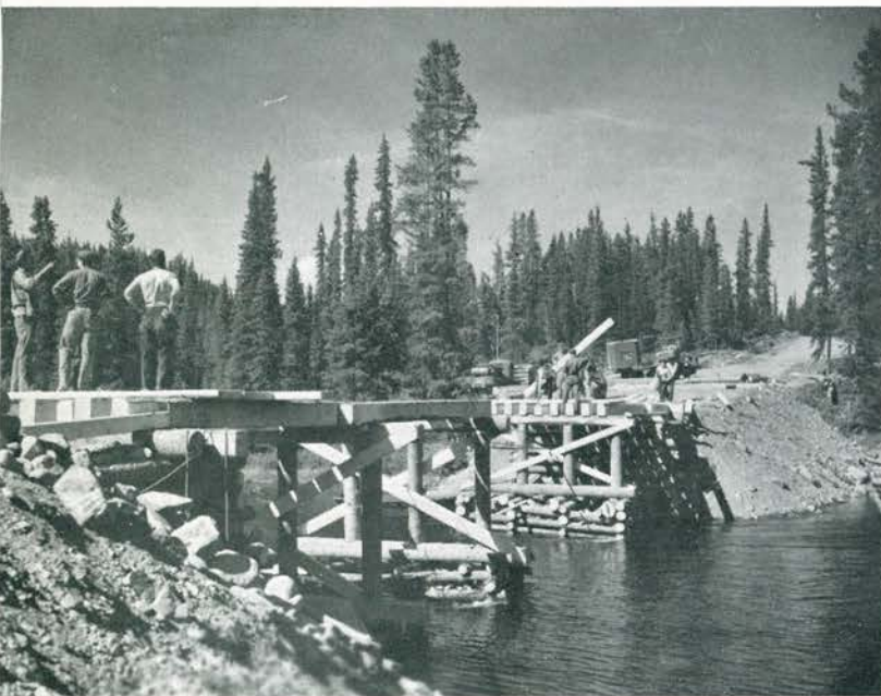
Only the center span stringers are yet to be placed as the Morley River bridge assumes shape. Flooring is already being laid.
