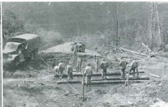
Company E building a small bridge over one of the numerous streams fed from melting snow on adjacent mountains.
