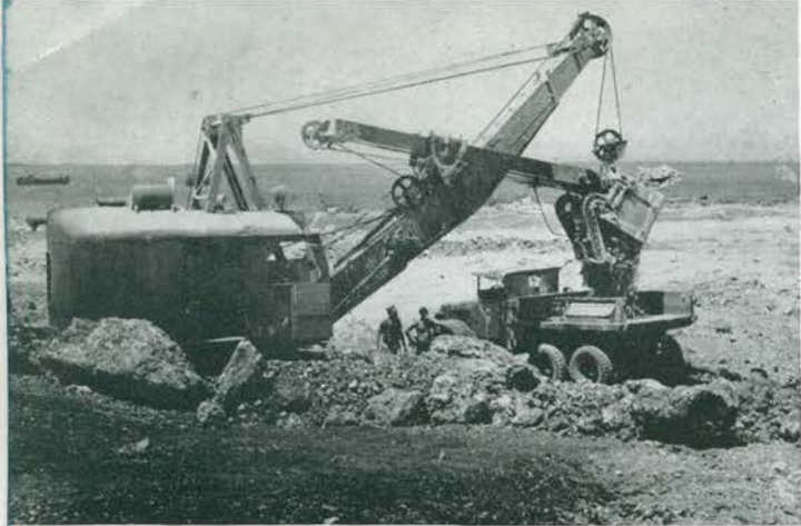
THE SHOVELS AND TRUCKS ARE KEPT BUSY BRINGING CORAL TO THE AIRFIELD
