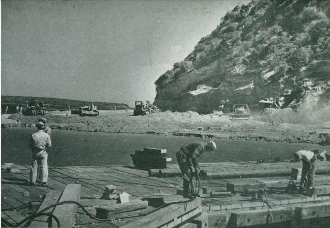
BY HAND AND ELECTRIC DRILL THE BOLTS SINK INTO THE TOUGH WOOD.
