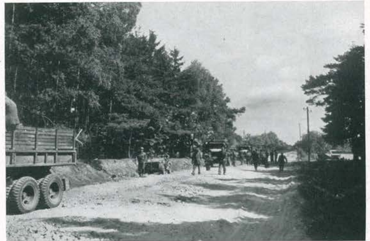
Main road between Hagenow and Schwerin, Germany being repaired by German PW's under the supervision of the 12th Combat Engineer Battalion. May, 1945.
