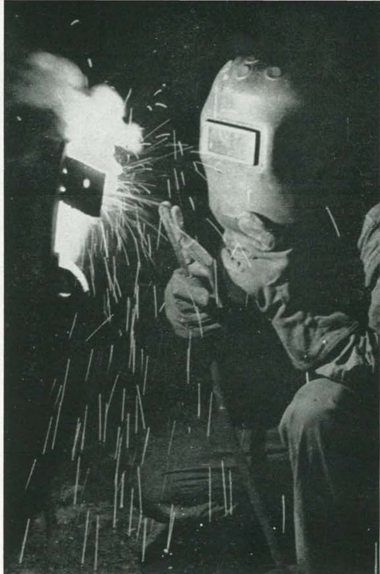
Upper right: A 28th Special welder, looking like a man from Mars in his mask, doing his work at night. The welders did a grand job in quickly adapting existing equipment to special circumstances.
