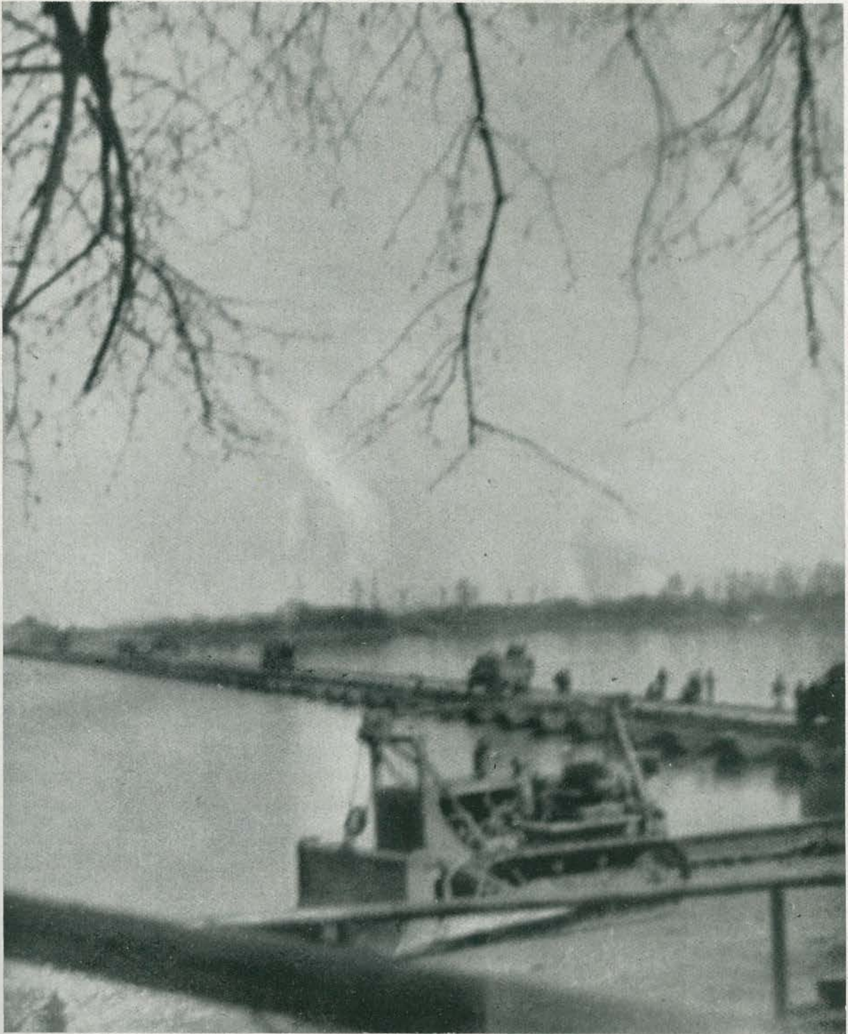
Pontoon bridge constructed by combat engineers. The bulldozer is invaluable for such operations as this and figures prominently in our march across Europe.
