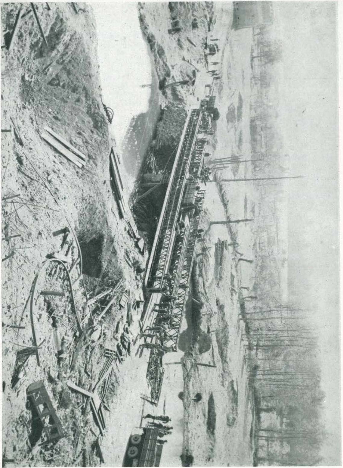
Enemy demolitions fail to impede our progress as engineers work with precision and skill.
