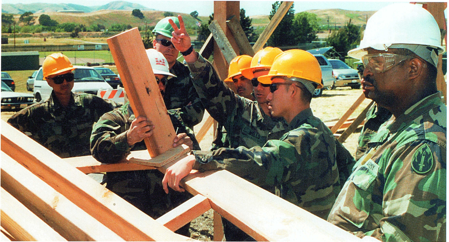
Soldiers from the 801st Engineer Company work at constructing a pavilion at Parks Reserve Forces Training Area. From left are, Sgt. Leland Ng, Staff Sgt. Frederick Jose, Staff Sgt.
