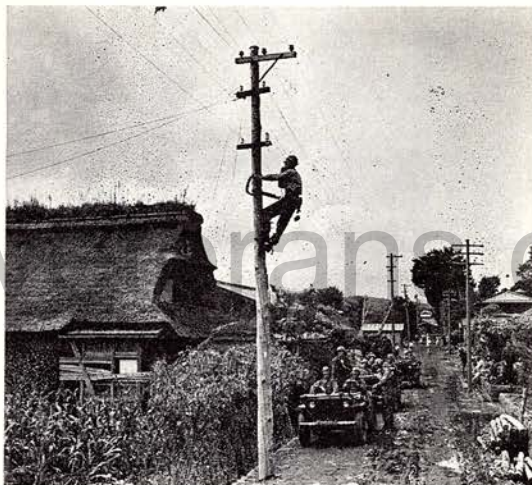
A lineman of the 13th Signal Company searches out a faulty line in the intricate telephone system composed of American and Japanese equipment connecting camps of the division.
