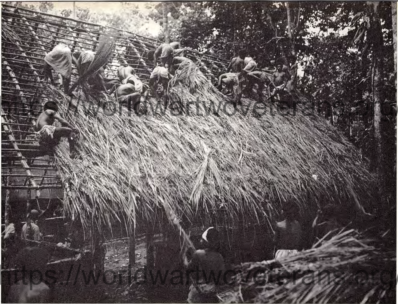
COMMAND POST PROJECT: Fuzzy-Wuzzies build a thatched roof structure for the Division command post at Goodenough
