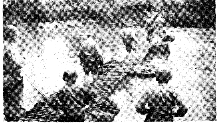
HERE THEY GO over the river on the bridge made from truck tarpaulins and logs. To demonstrate their faith in their own work, all the men who worked on the project crossed the bridge they'd built.
